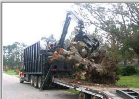
Hazardous Stump Removal
