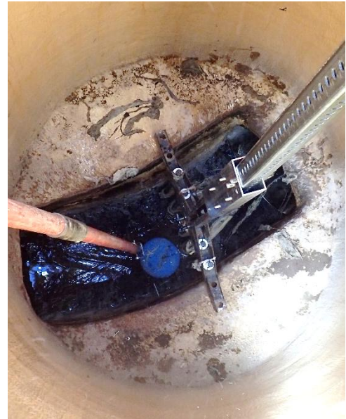
Figure 3. Example of Bar Screen Extraction of the SmartBall Tool
